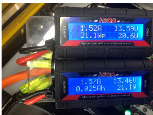
Figure 17 Wattmeters used with the battery chargers to monitor energy consumption and recharge compared to battery capacities.
